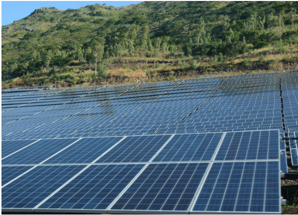
Solar farm in Mauritius
