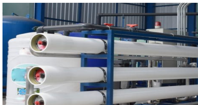
Desalination Plant in Rodrigues
